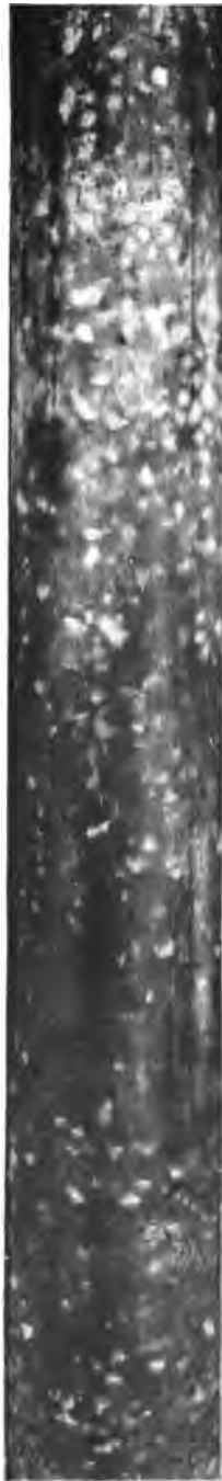
CONCRETE COLUMN, 1 : 2 : 4 MIXTURE. SPOTTED APPEARANCE, WHEN THREE DAYS OLD, ATTRIBUTED TO IRREGULAR DISTRIBUTION OF STONE AGGREGATE; EARLY DRYING OF MORTAR OVER THE STONE.
